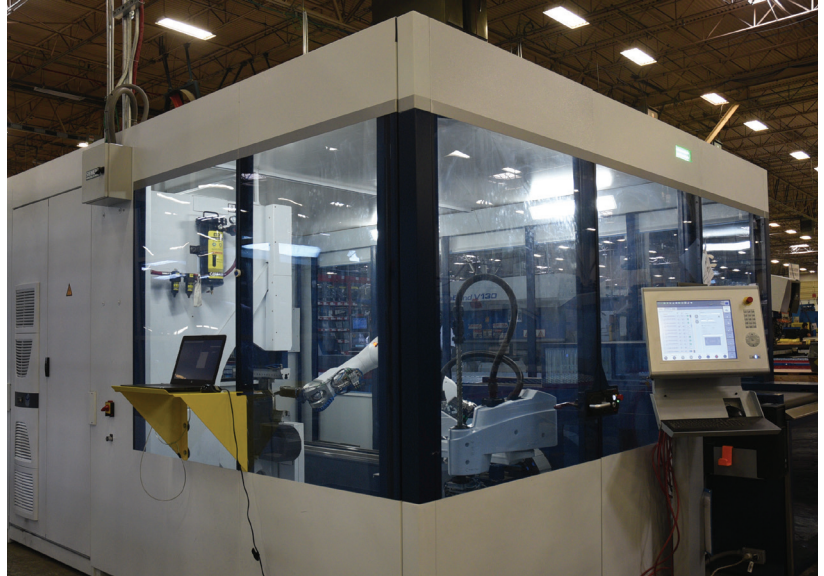
Figure 4: The SCALANCE networking components throughout the facility and in the enclosure in the upper left, support the automation devices.
