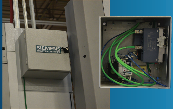
Figure 1: One of 38 SC ALANCE SC636-2C firewalls securing the automation network
