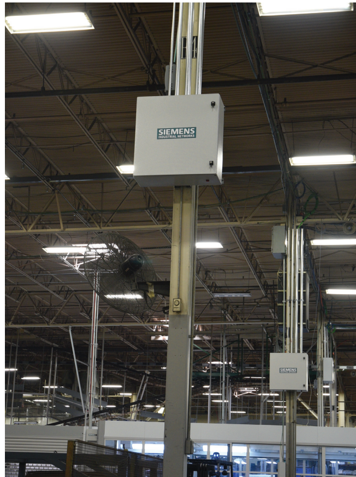
Figure 2: Enclosures house a SCALANCE X416-4C to establish the network backbone with a ring
