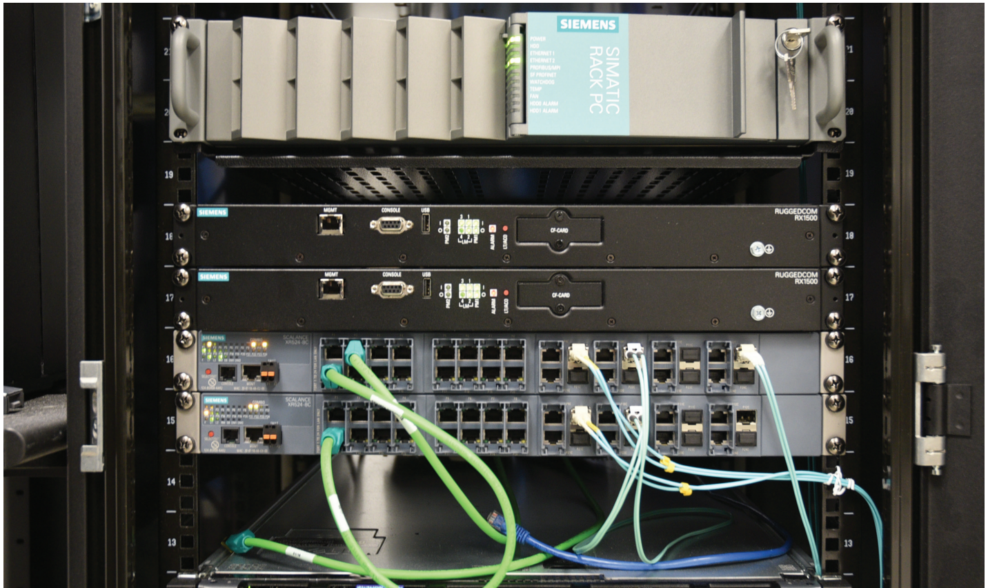
Figure 3: SCALANCE XR524-8C Layer 3 switches on the server rack as part of IT / OT collaboration
