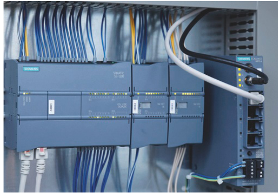
Always well connected: SCALANCE M mobile wireless routers from Siemens ensure reliable transmission of data for remote control of the double sluice gates despite difficult cellular network coverage.
