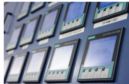
23 measuring devices from Siemens' 7KM PAC series measure values such as current, heating, cooling, or compressed air
