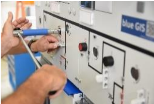
Image 6: Siemens blue GIS 8DJH switchgear
