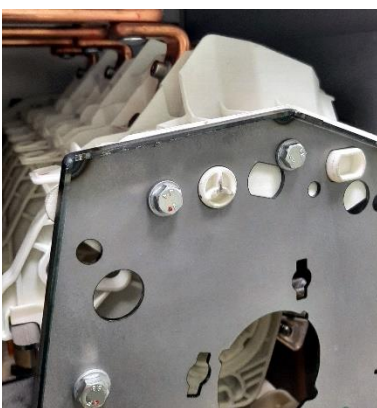
Image 3: blue Switch disconnecter with vacuum interrupter
