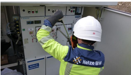
Image 4: Substation at Netze BW GmbH
