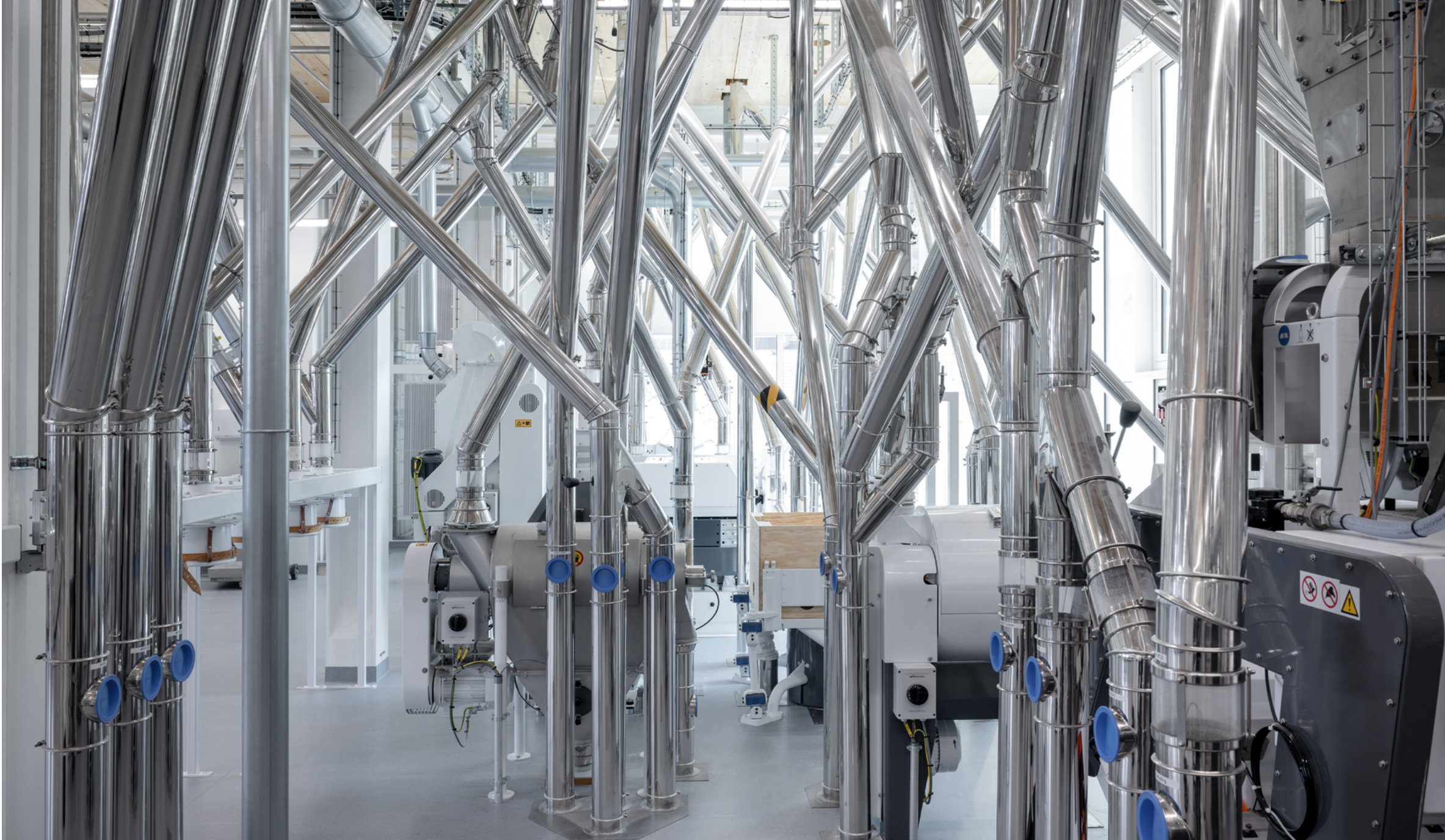
High-end mill construction: Bühler relies on Siemens for automation in its state-of-the-art Grain Innovation Center.
