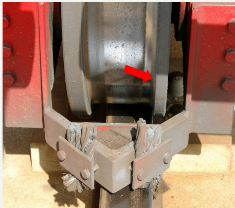
High wear and tear of crane wheels due to frequent contact of wheel flange against the rail.
