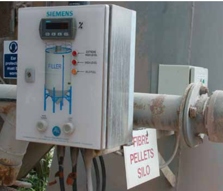
SITRANS RD200 remote display, connected to this custom-built panel, shows level percentages in the fibre pellet storage vessel.
