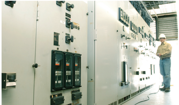
After: Following the field modification, the breaker can be racked in and out while the operator stands outside of the arc flash zone.
