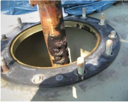
Defective bushing element and bushing pin
