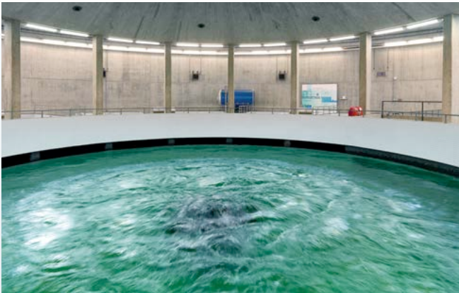
Water pumping station
