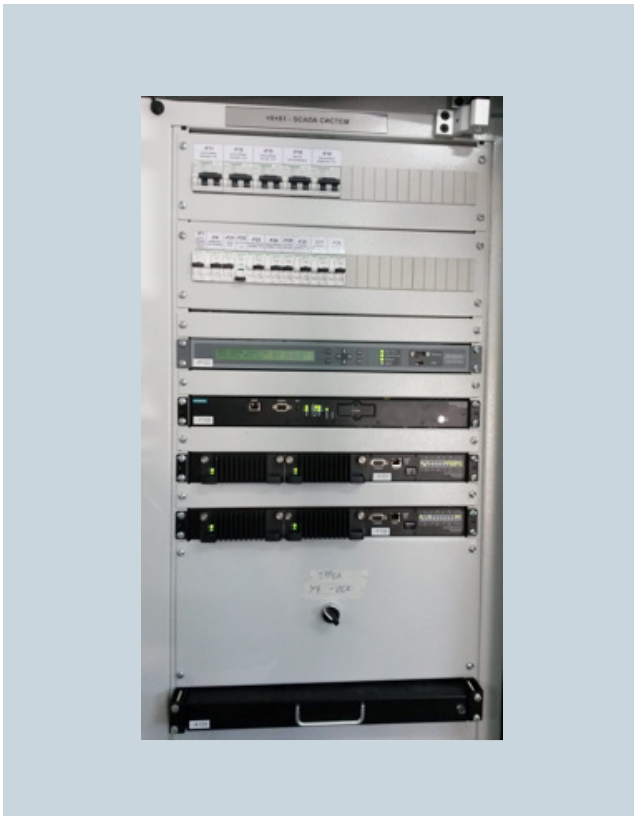
The RUGGEDCOM RSG2488 – a reliable, 28-port high-performance switch is used in a communications network for substation protection and automation and SCADA monitoring and control.
