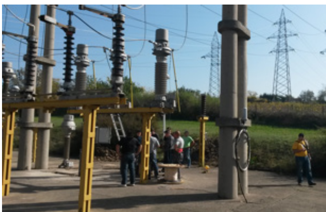
Remote monitoring, control and automation of nine transmission substations posed some challenges to the Macedonian transmission operator.
