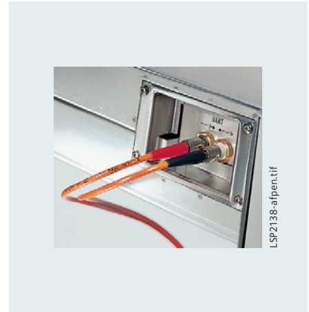
Fig. 5/36 View from below showing system interface (SCADA) with FO connection (for remote communications)
