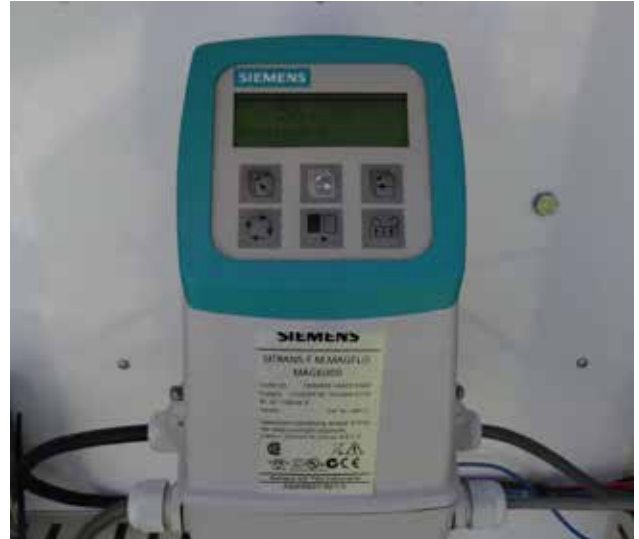
SITRANS F M MAG 6000 transmitter remotely connected to the 66-inch SITRANS F M MAG 5100 W flow meter sensor.
