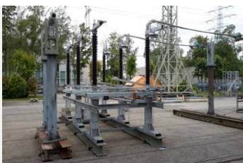
Center break disconnector 3DN1
