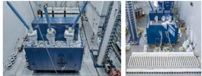
Power transformer with ester insulation and heat exchanging device in the testfield
