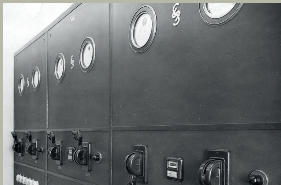
A traction current converter plant. Hotel Imperial, Karlovy Vary
