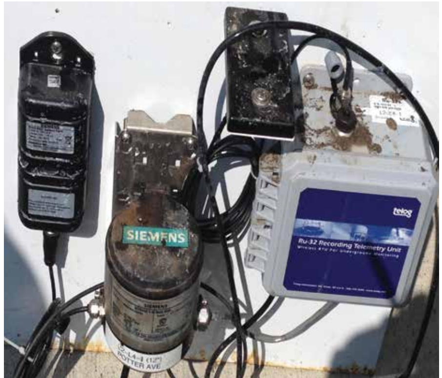
Figure 4 Flow transmitter, battery, data logger and modem
