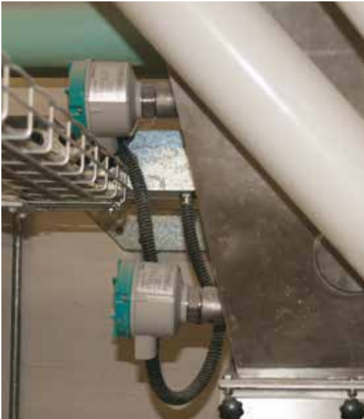
SITRANS LPS200 level paddle switches monitor high and low levels in the gluten hopper.
