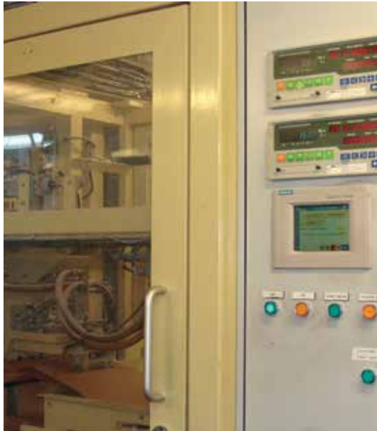
A SIMATIC HMI panel monitors the company's finished flour bagging operations and can be customized to the bagging operations.
