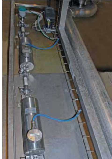
The field test setup, consisting of two existing Siemens Coriolis meters and the new SITRANS FC330.
