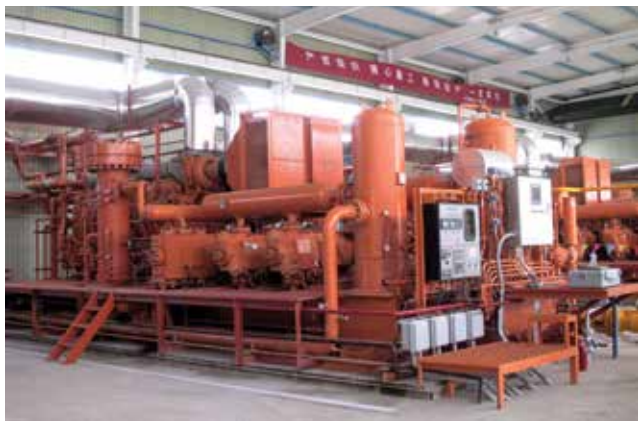
Six-throw HOS compressor installed in China.
