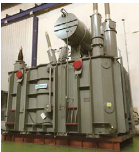
500-kV single-phase autotransformer in the test bay
