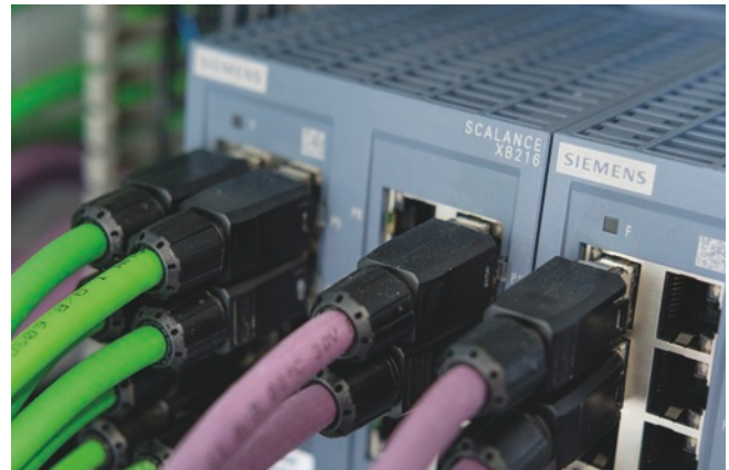
Color-coding is used to keep the overview between realtime automation (green cables) and IT-communication (pink cables)
