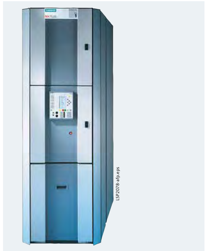
Fig. 5/68 NX PLUS panel (gas-insulated)
