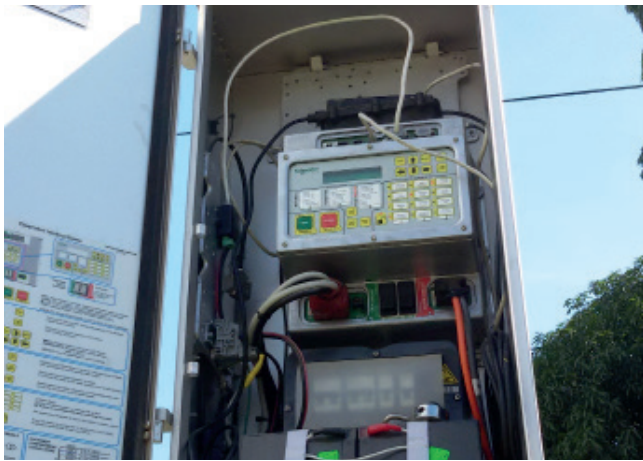
Wide area network visualization and substation automation (SCADA for PLCs/RTUs/reclosers)
