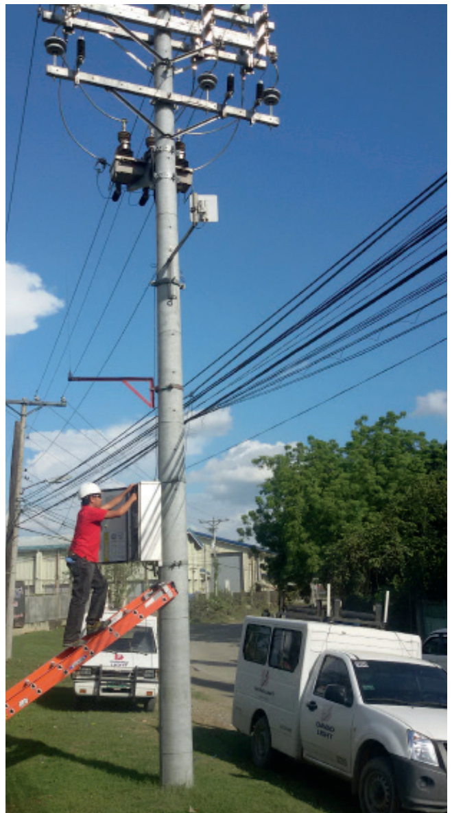
Demand response, remote disconnection
