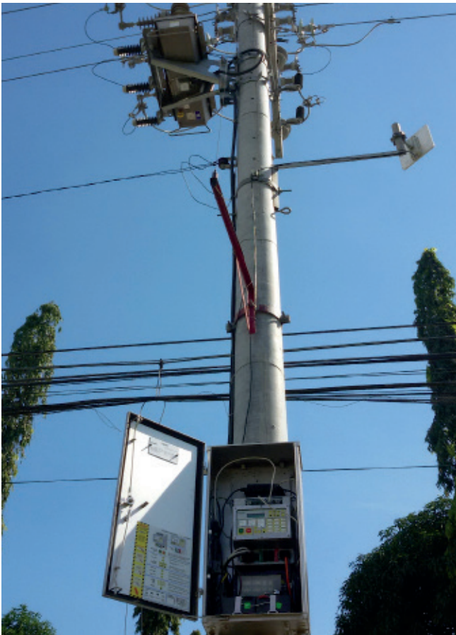
Wide area network visualization and substation automation (SCADA for PLCs/RTUs/reclosers)
