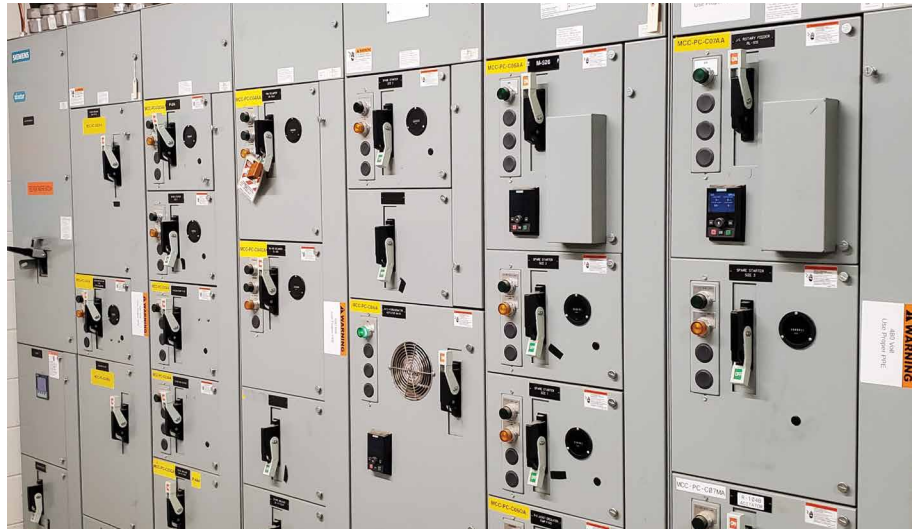
TIASTAR Motor Control Centers (MCCs) monitor and manage motor operation, energy consumption and power quality throughout the site. SINAMICS Variable Frequency Drives are connected to the MCCs for more precise control of motor speeds.
