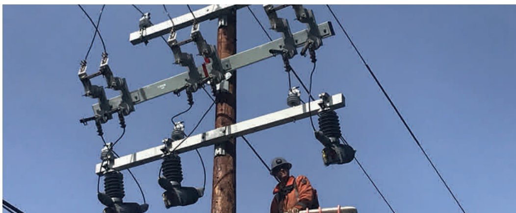
B-2 bypass assembly installed with CMR compact modular reclosers
