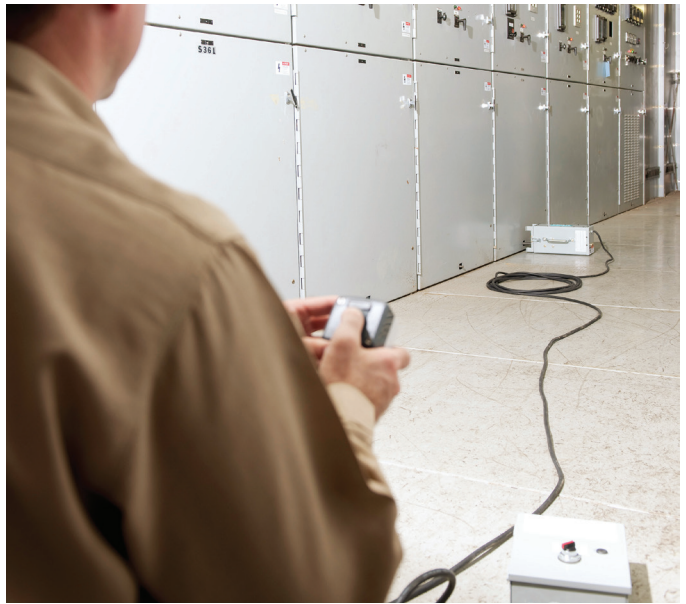
After: Following the field modification, the breaker can be racked in and out while the operator stands outside of the arc flash zone.
