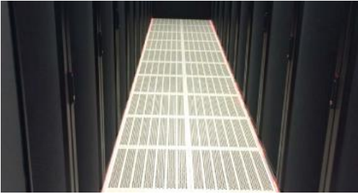
WIEN IT – FLORIDA | Data Center
