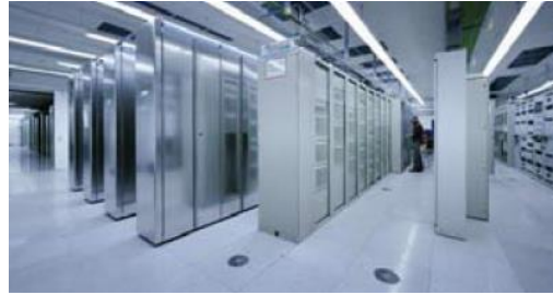
INTERXION, WIEN | Data Center
