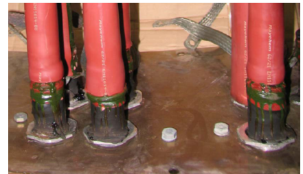
Figure 2: Thermal damage to cables
