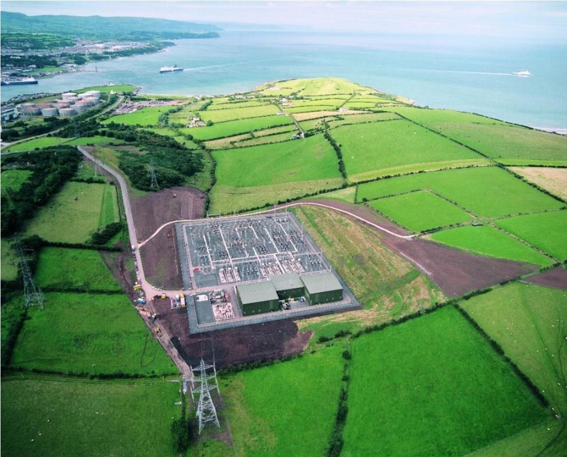
HVDC converter station in Ballycronan More, Northern Ireland.
