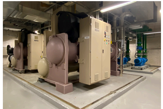
Advanced energy efficiency control for both chilled water pump and cooling water pump uses high-precision sensors and monitoring system to control the entire chiller system.
