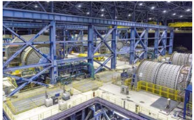
Figure 4: Two SAG Mills 24MW each and Two Ball Mills 16.4 MW each with Gearless Mill Drives
