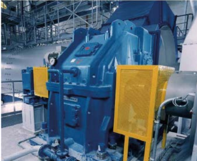
Figure 6: 2500 kW multi stage gear unit for a ball mill in a silver mine
