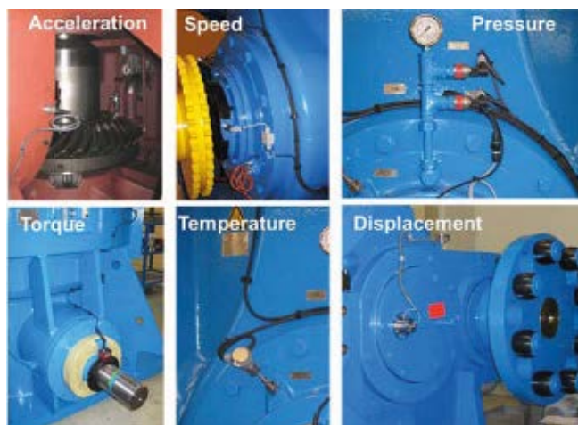
Figure 5: Examples of sensors installed in a large gearbox unit for a grinding mill
