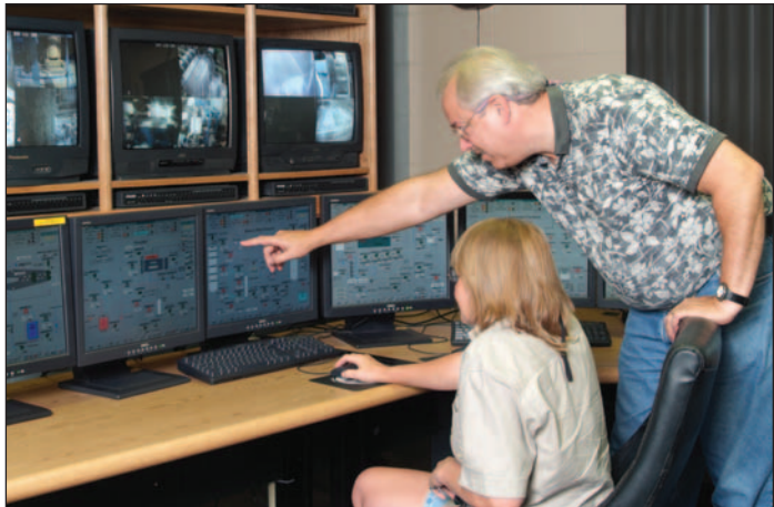
MRC’s decade old hardware forms the backbone of the new Siemens system.
