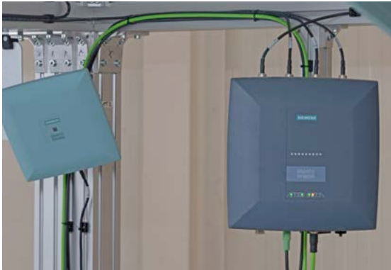
Core components of the RFID solution are a SIMATIC RF680R UHF reader (center) and up to four RF680A antennas with switchable polarization for best reading results under all environmental conditions.
