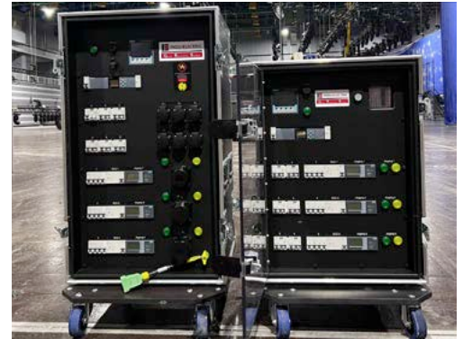
Concert distribution board with residual current monitoring of each socket outlet circuit via SENTRON 5SL6016-7MF miniature circuit breakers with RCM and power monitoring function – and with RCD protection of the sockets via SENTRON 5SV3 residual current protective devices and compact SENTRON 5SV1 RCBO (residual current circuit breaker with overcurrent protection).
