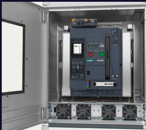
Cooling system with fans underneath the SENTRON 3WA air circuit breaker
