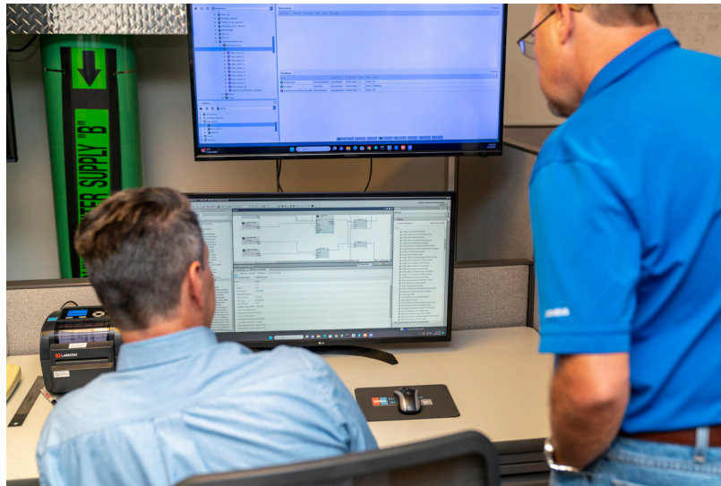
Reviewing HVAC equipment data at Colorado Springs data center
