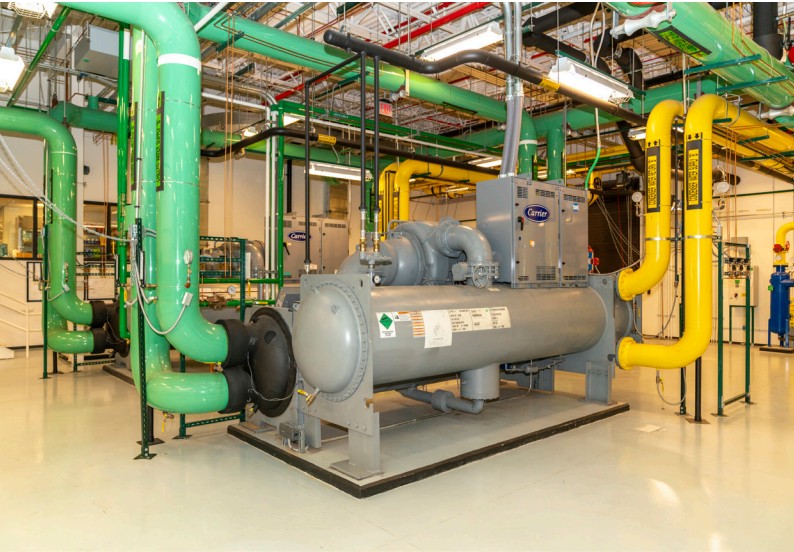
One of four chillers controlled by Siemens Desigo PXC controllers
