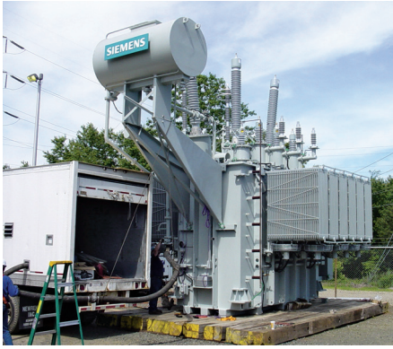
Transformer oil processing
