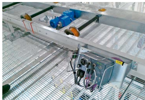
SIRIUS M200D motor starter are used at SEAT in Spain
