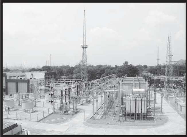
Siemens commissioned the 400 kV Synchronous Compensator (STATCOM) solutions at PGCIL's substation in Rourkela. The STATCOM solution provides optimal grid stabilization technology. The equipment has been manufactured at Siemens Ltd.'s manufacturing plant in Goa.
