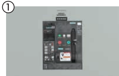
1 Main generator breaker key interlocked with normal main breaker (UL489 2000A WL pictured)
