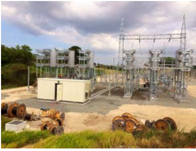
New Control Enclosure at Panama Substation
