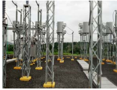
New 115kV Capacitor Bank at Substation
