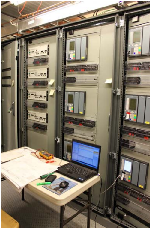
Testing of New Control Enclosure Relays
