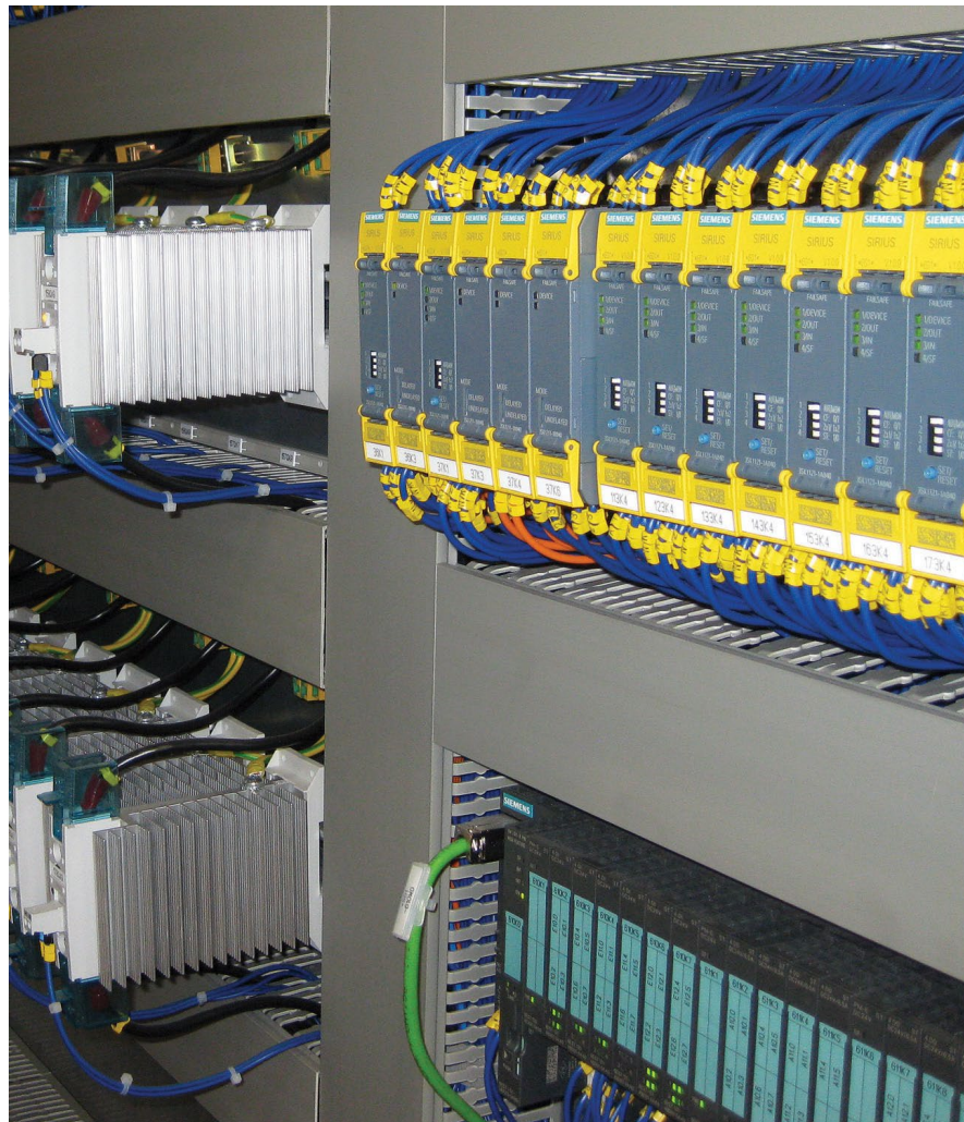
Figure 1 The monitoring and control scheme for these heat-treatment furnaces feature multiple IO-Link masters per furnace, located on the ET 200S distributed I/O from Siemens and connected with the controller via PROFINET.
