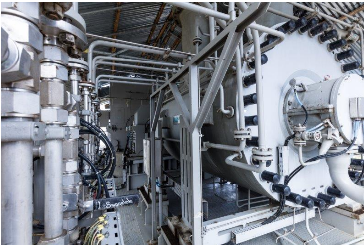
Above: Boil-off gas compressor.
