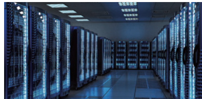
西门子变压器应用于国内外大型数据中心 SIEMENS transformers in several large data centers all over the world.
