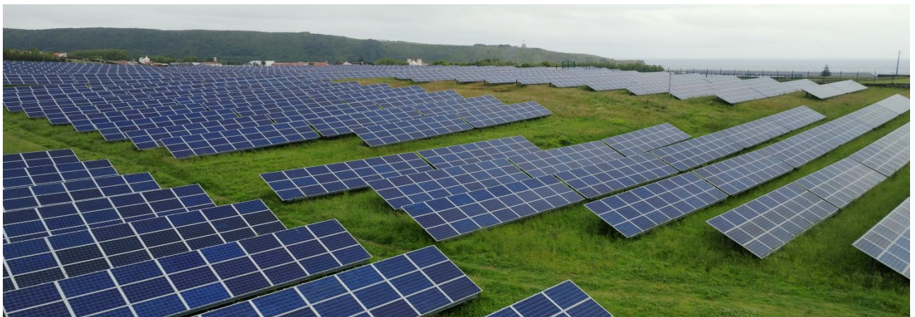
Figure 2: Ground-mounted photovoltaic plant
