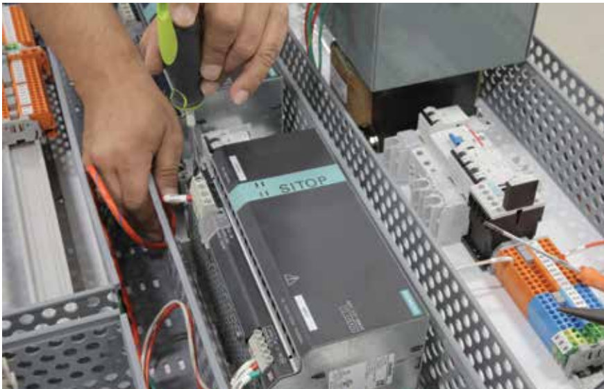
Flexible set-up permits on-the-fly adaptation of control hardware, when changes are required or subsequent iterations of a machine are produced.
