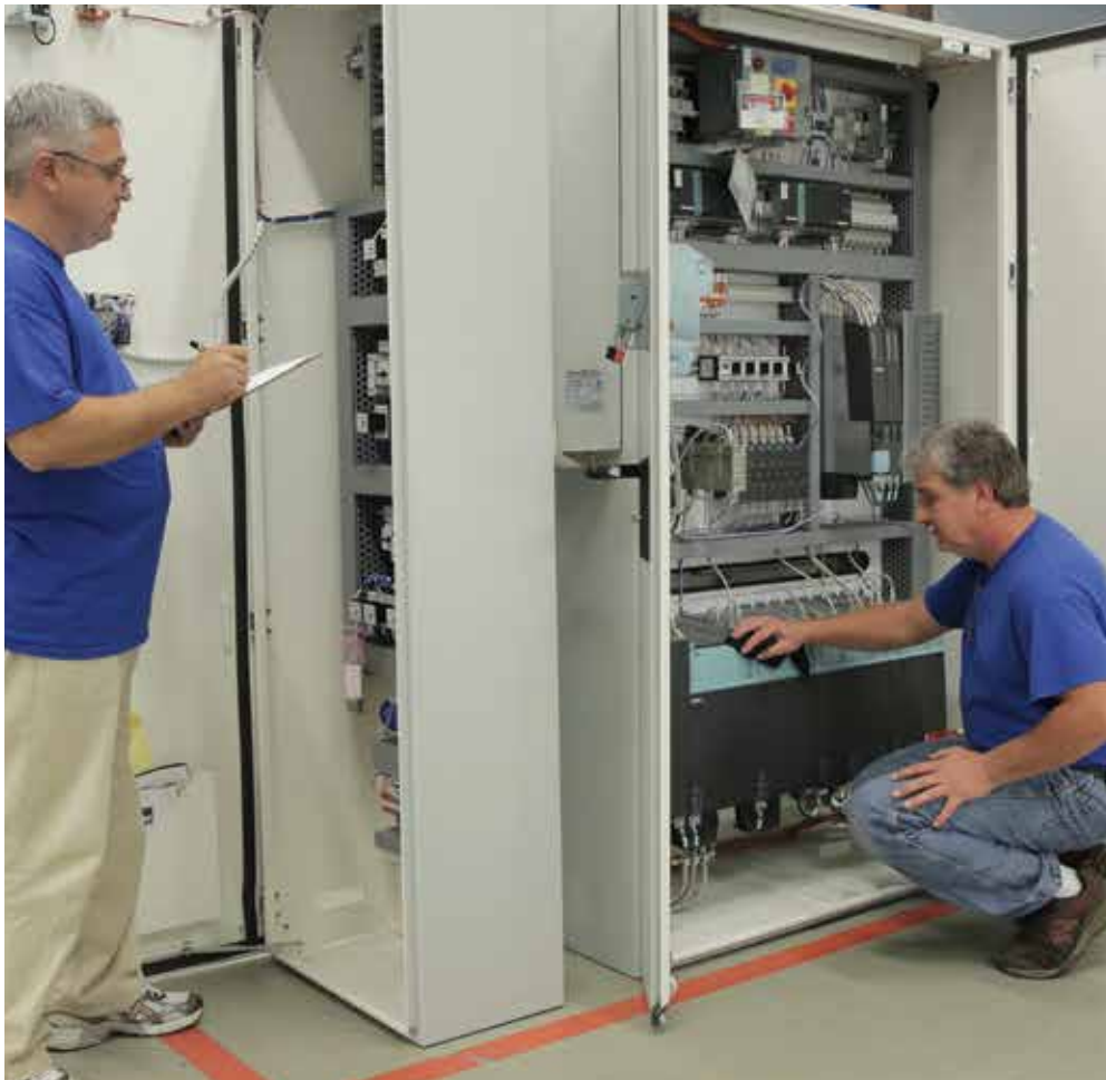
Simplified designs are made possible by the expertise of custom panel builders, who bring experience in component clustering, footprint and enclosure space utilization to the task.
