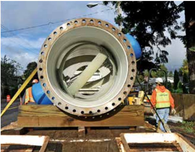
The installation of the system at SW 147th Avenue and Powell in Portland, Oregon.
