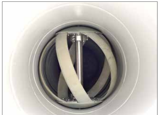
Siemens motors are powered by the turbulent flow of the water through the municipal water line. The energy is captured and transmitted to the PGE grid for powering the local community.
