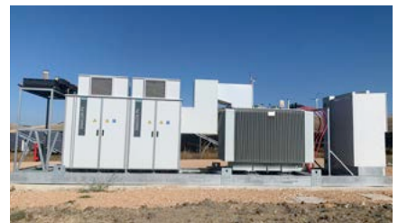
Troia energy site
