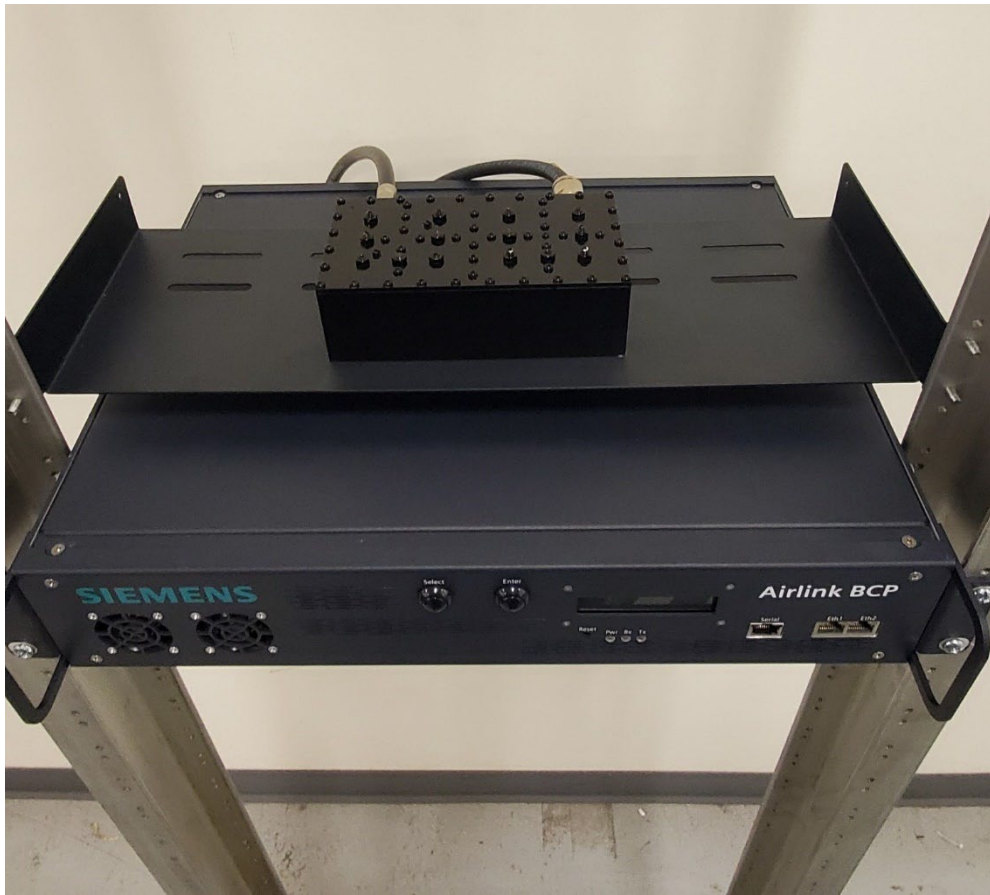
Figure 4-6 Duplexer and Airlink BCP Front Views when Mounted to Rack
